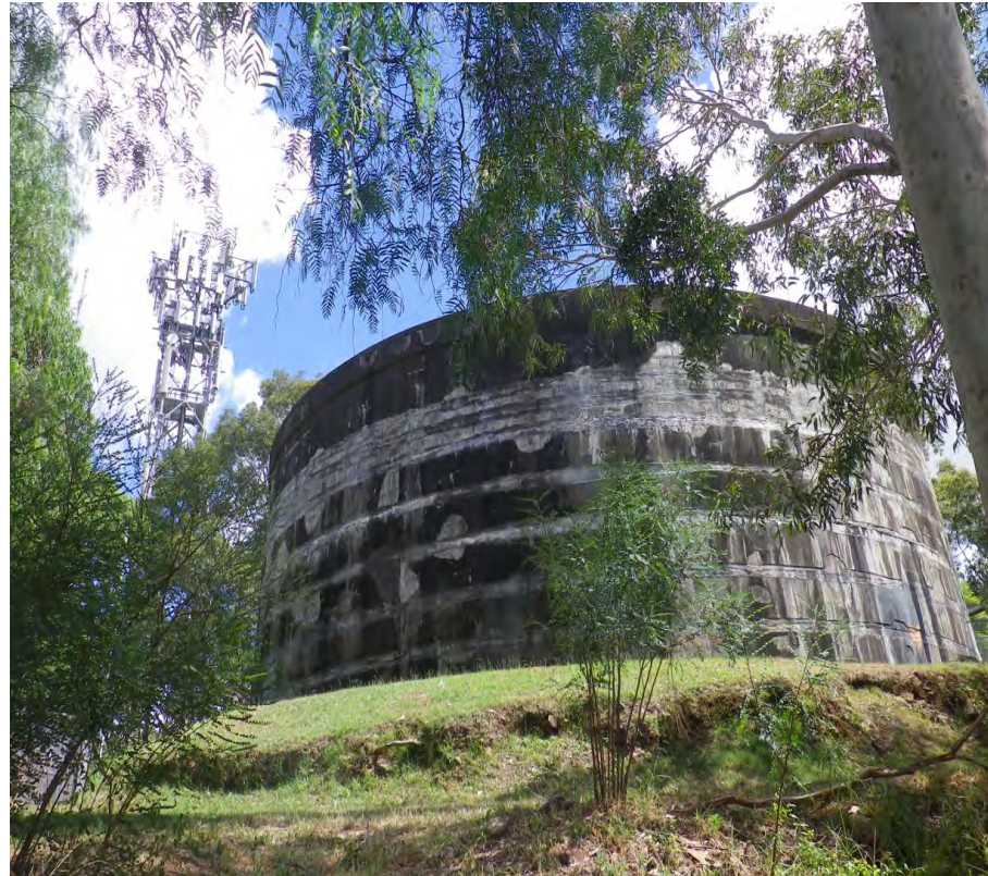
Reservoir water tank
